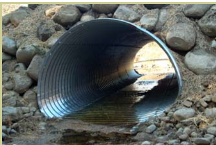
This box arch culvert was installed on the Penobscot Nation’s Land to replace a failed double culvert system.
