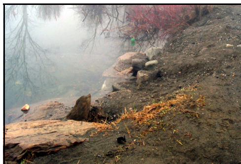
An example of an eroded road bank.
