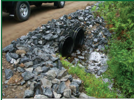
An example of a properly installed and armored culvert in the Sebasticook Watershed.
