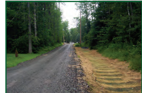
A properly constructed road ditch will require less maintenance and save money in the long run.
