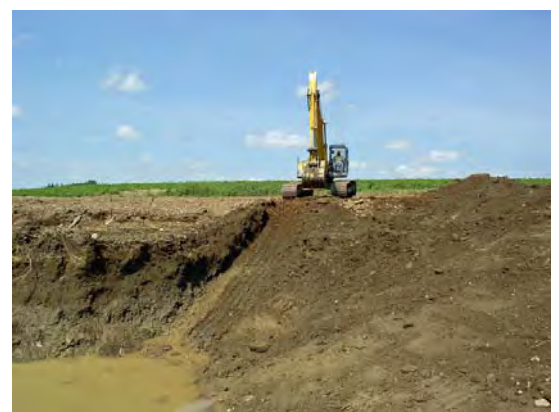
This excavator is creating the berm that will hold the water for the pond.
