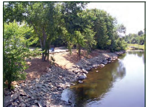
Here is the same section of the river bank shown above with several stabilization practices installed including rock rip-rap and excelsior matting with grass seed.
