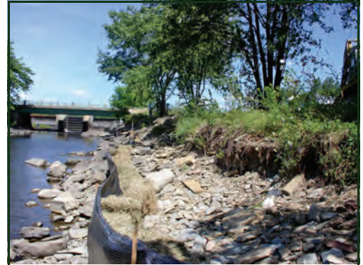
This is just one example of the severely eroded river banks on the East Branch Sebasticook River directly below Sebasticook Lake.
